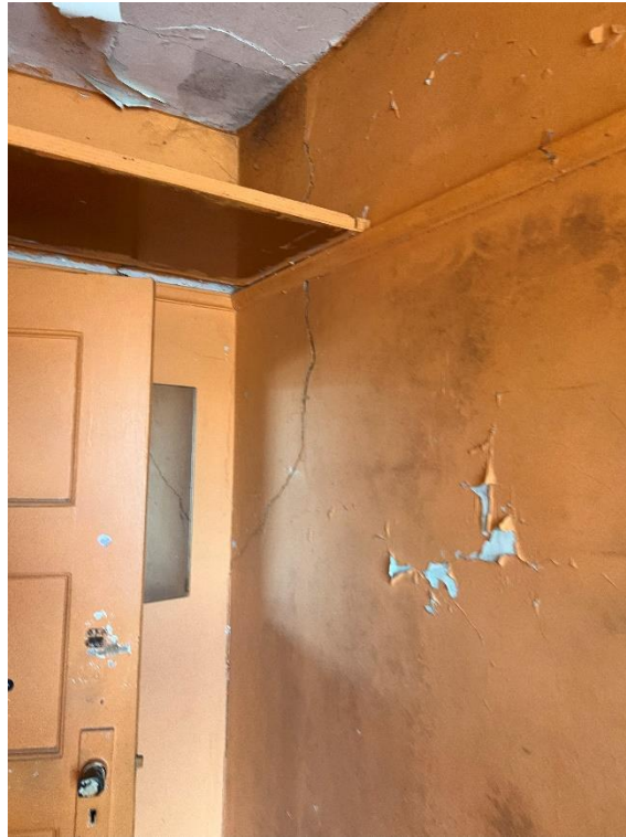
Photo 19 – Crack in the side elevation wall – front room at 2 nd floor level
