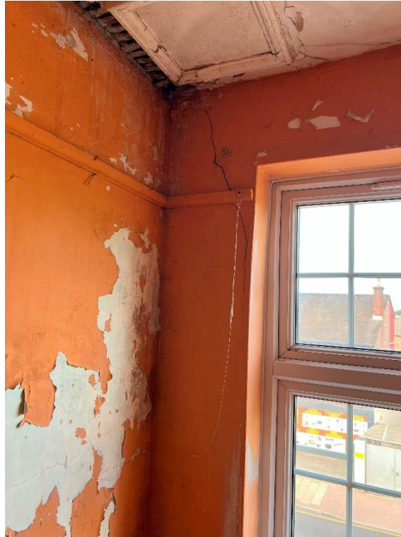
Photo 17 – View from inside at 1 st floor level looking out of front elevation – Note crack to top of window
