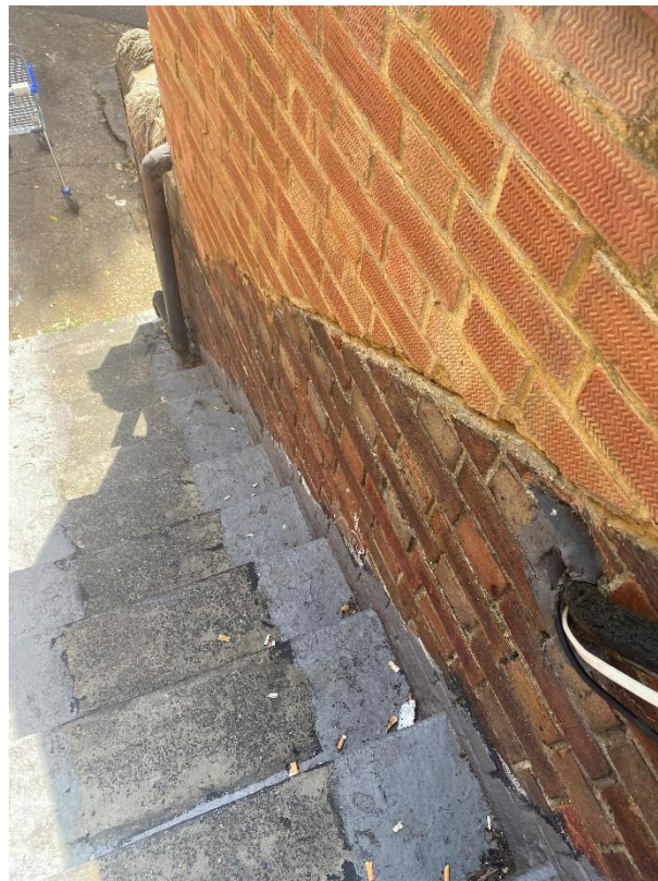
Photo 4 – Close-up on rear access steps – Rear Extension constructed on top of older brickwork
