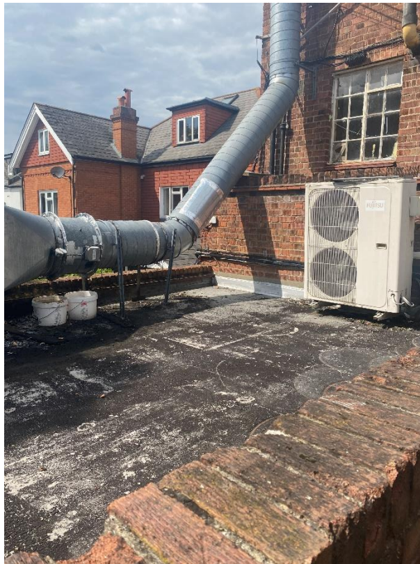
Photo 6 – Ventilation shaft and mechanical equipment
