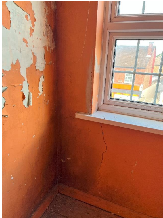
Photo 18 – Note crack at the bottom of the window
