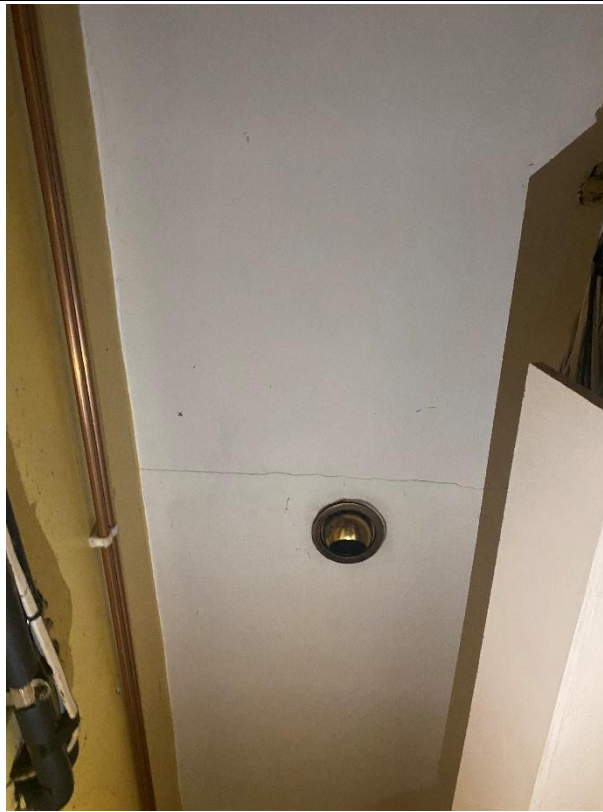
Photo 21 – Ceiling crack in the ground floor corridor
