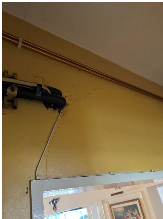
Photo 20 – Crack above the door opening
