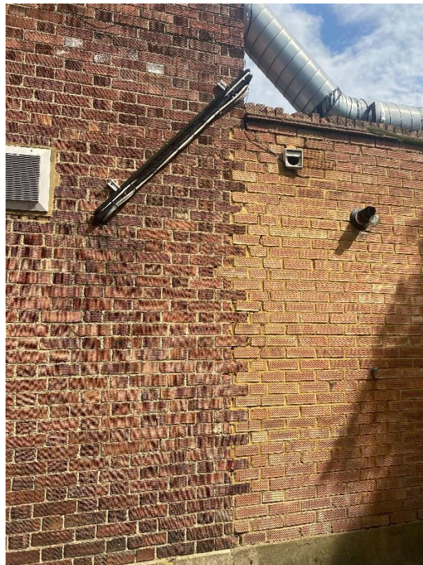
Photo 10 – Close-up on Photo 9 showing cracks at the junction
